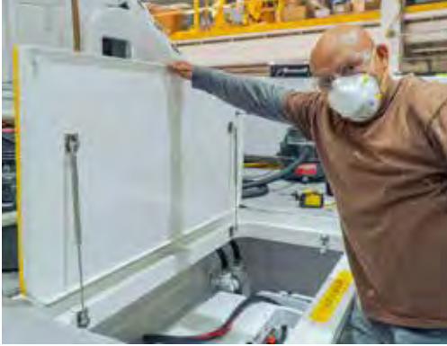
Inocente Silva completes the installation of a pair of stainless steel gas pistons in a cockpit hatch.
