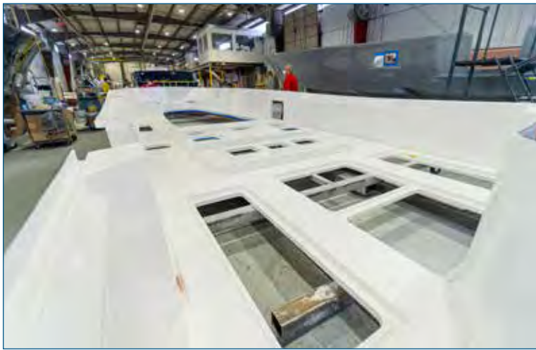
The deck liner with its integrated hatch openings is ready to be installed in the hull.
