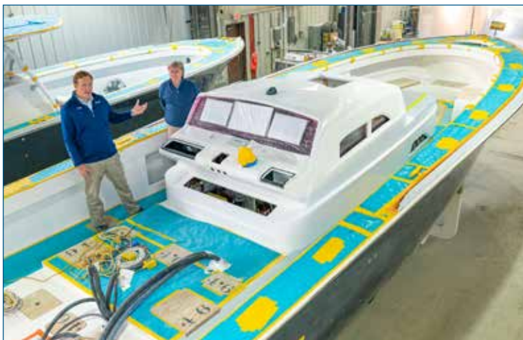
With the console installed and the machinery room and cabin taking shape, Viking Mullica General Manager John Leek IV and President and CEO Pat Healey film a video update of the build process.
