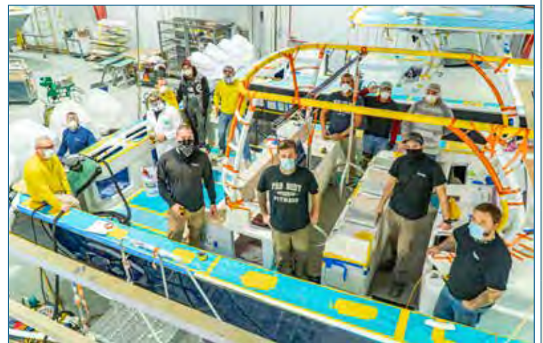
With the seating modules and hardtop frame now in place, Viking Mullica shipwrights gather for a quick photo before getting back at it.
