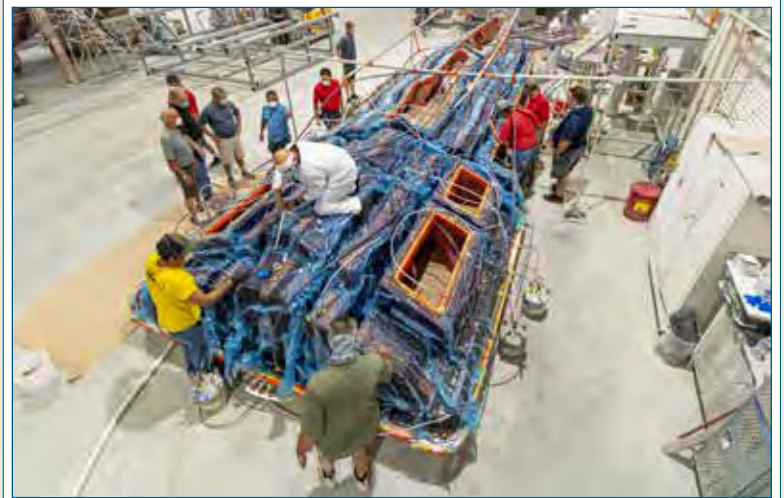
All hands on deck for the resin infusion of the structural stringer grid.
